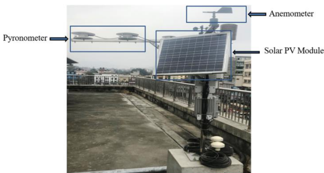
Data logger at Singhdarbar, K3 substation, Kathmandu Nepal
